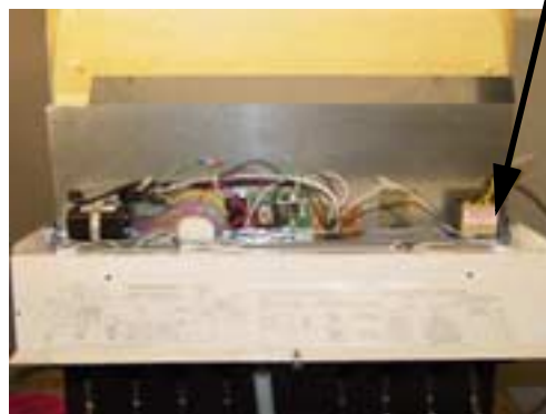
FIGURE 29. Electrical Box 2x Single Transformer
